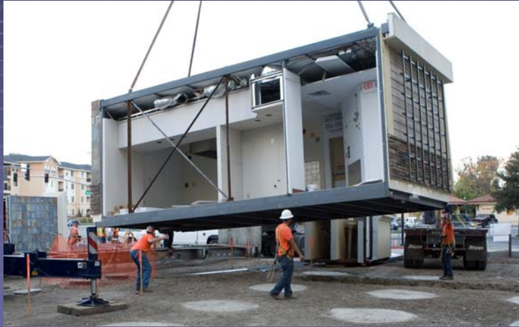
Modular Being Installed, Lifted from Above, All Interior Finishes and Fixtures Completed
