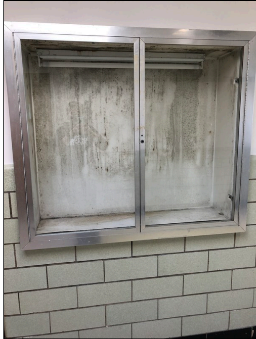
1 - Display case in hallway with visible microbial growth
