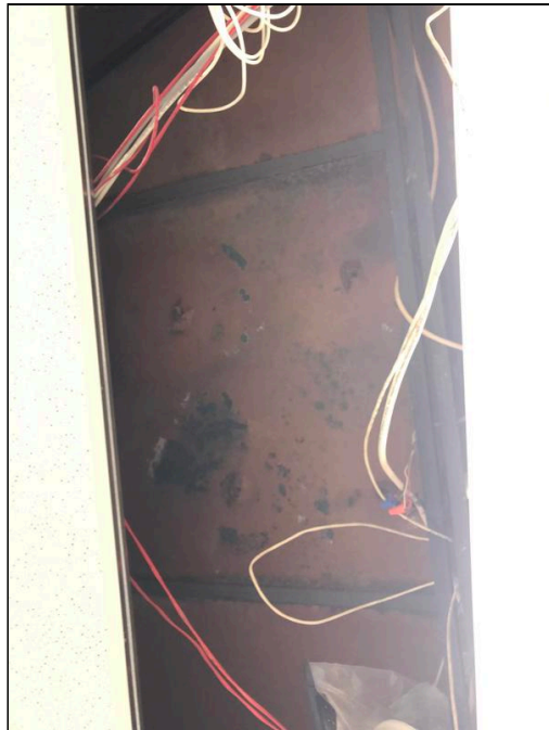
2 - Visible microbial growth above drop ceiling in the hallway
